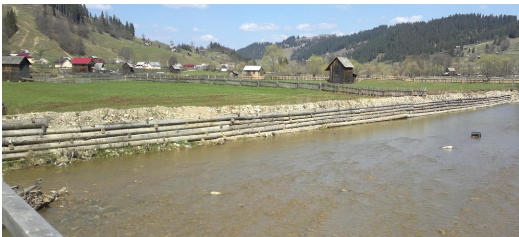
Figure 3: Crib wall bank protection on Moldovita river in straight zone
